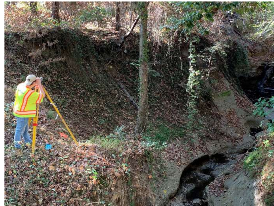
SEVERELY ERODED STREAMBANK
