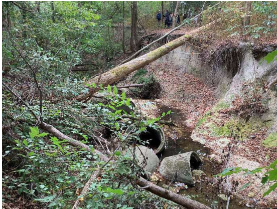
DAMAGED 60" PIPE OUTFALL
